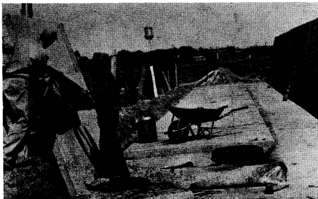
Fig. 15.—Putting side walls, formed in segments of reinforced concrete, in place for the experimental above-ground trench silo.
